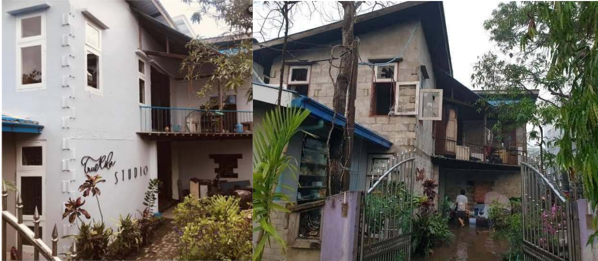
Figure 58: Before and after damaged images on True Colour Studio, set alight in the early hours of March 17, 2021.
