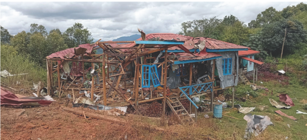
Figure 34: Images shared on the day of the alleged airstrike appear to show structural damage to the rear of Kuafo Baptist Church (top), a large crater in the ground behind the church (middle) and a destroyed residential building (bottom). This footage has been compared with a video also claiming to show the aftermath of the incident (see Figure 33) and has been geolocated by Myanmar Witness (source: Khit Thit Media ).
