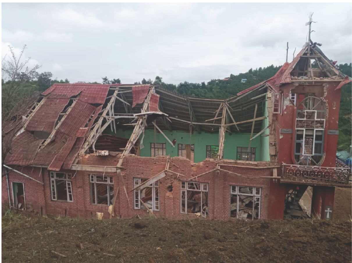
Figure 30: Footage shows a large hole in the roof of the church, in addition to structural damage to the towers and brickwork (sources: The Chin Journal , warning: graphic link; personal Facebook account, redacted due to privacy concerns).
