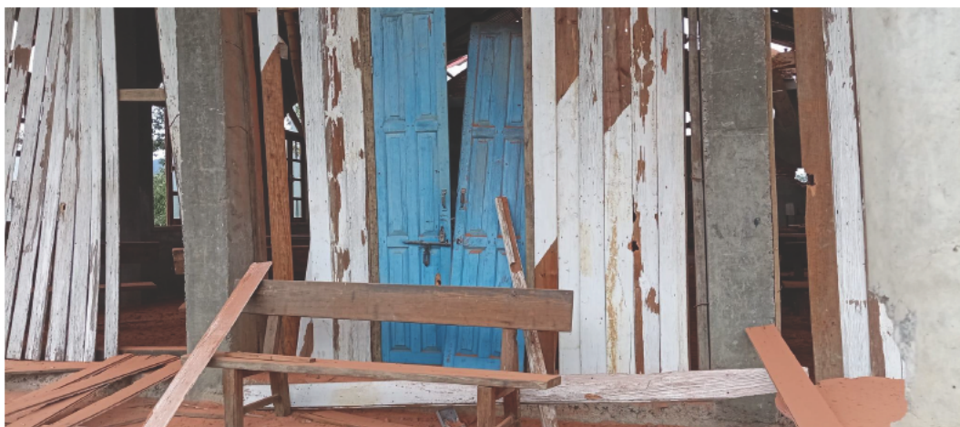
Figure 31: Imagery from the claimed airstrike on Khuafo. Damage to the interior of Khuafo Baptist Church (top), along with damage to the front door and walls of the church (bottom) (source: Khit Thit Media ).
