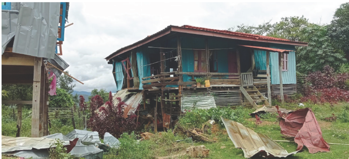
Figure 36: UGC showing damage to a residential building in Khuafu, geolocated by Myanmar Witness [22.752099, 93.425127] (source: Khit Thit Media ).
