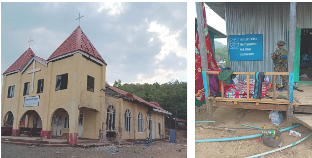
Figure 19: Footage shared by The Chin Journal shows extensive damage to Malsawm Baptist Church (left), which can be identified by the sign above its main entrance. Additional UGC shows the aftermath of the alleged military occupation of Believers Church Malsawm (right) (source: The Chin Journal ; personal Facebook account, redacted due to privacy concerns).
