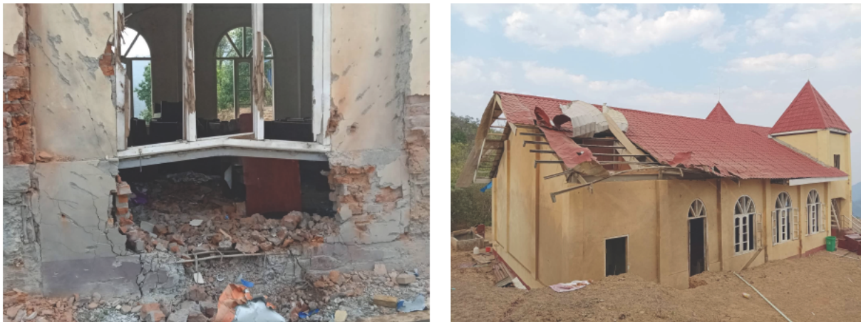
Figure 21: Geolocated UGC showing structural damage to the exterior wall and roof of Malsawm Baptist Church (sources: Chin Human Rights Organization ; personal Facebook account, redacted due to privacy concerns).
