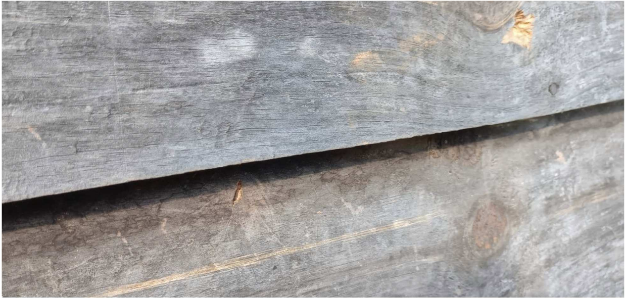
Figure 13: Side-on images of the damage, showing two entry penetration marks, exposing new wood, with one being higher and larger than the other.
