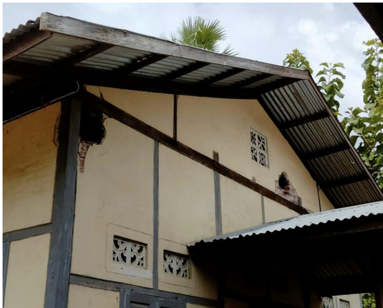
Figure 33: Outside building damage in Let Yet Kone village, showing large gaps allegedly from airstrikes on 16 September 2022 (Source: Private).
