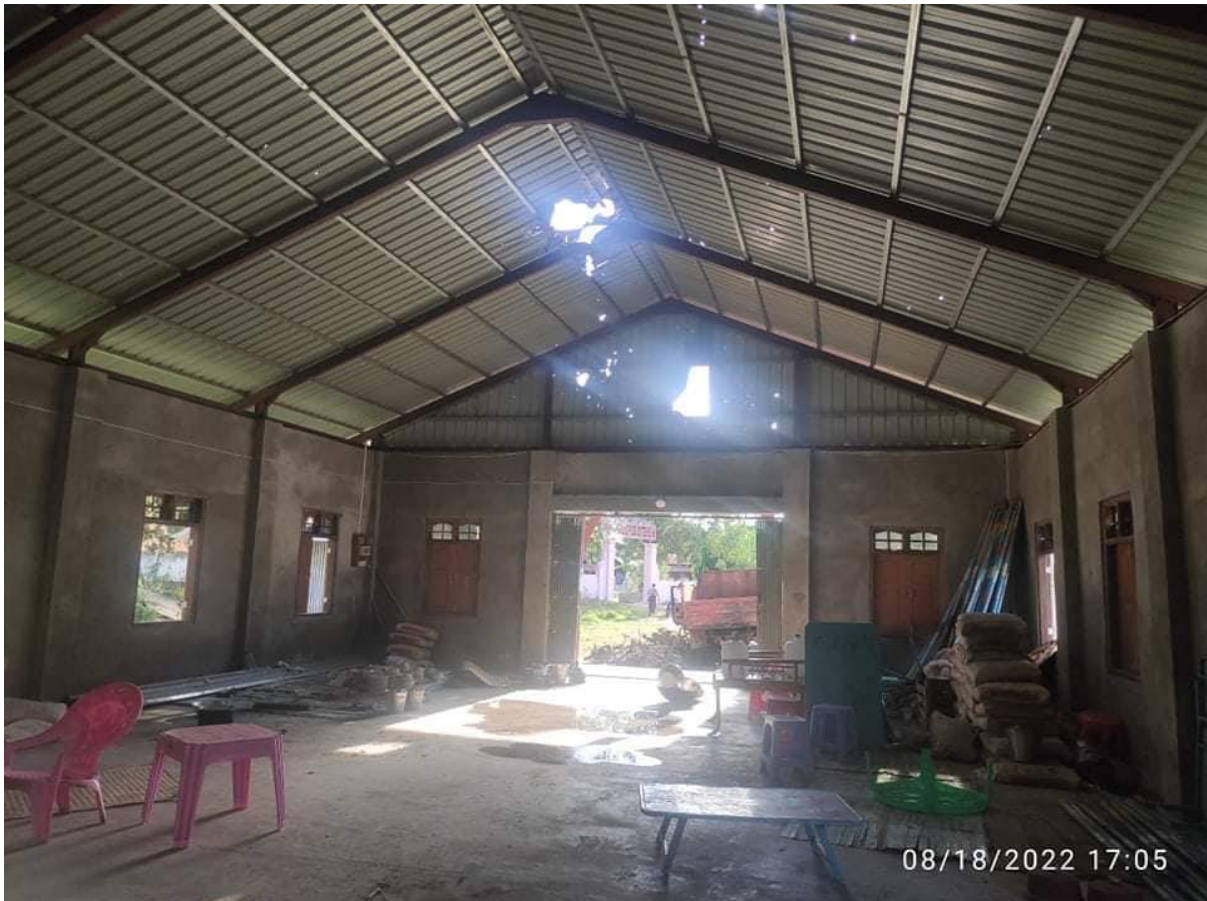
Figure 15: The red roofed building, located at 22.073185, 94.789669, demonstrates damage to the building's roof. (Source: Private).
