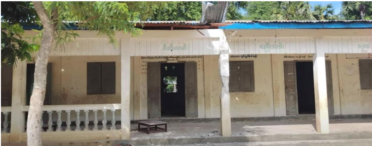
Figure 32: Several different angles of destruction of one building identified by Myanmar Witness to be located at 22.679200, 95.400131 (Source: Khit Thit Media ).
