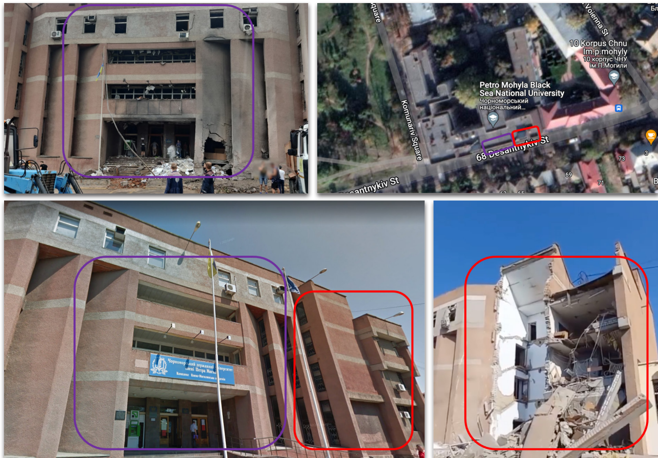
Figure 15: The damaged entrance of Petro Mohyla Black Sea National University in Mykolaiv [46.971667, 32.015109].
