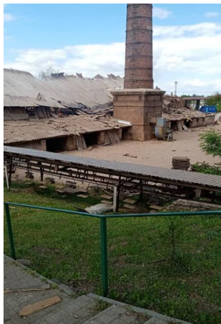
Figure 9: A screenshot taken on 14 June, showing a destroyed brick factory as a result of Russian shelling; geolocated to 49.799232, 24.905078.
