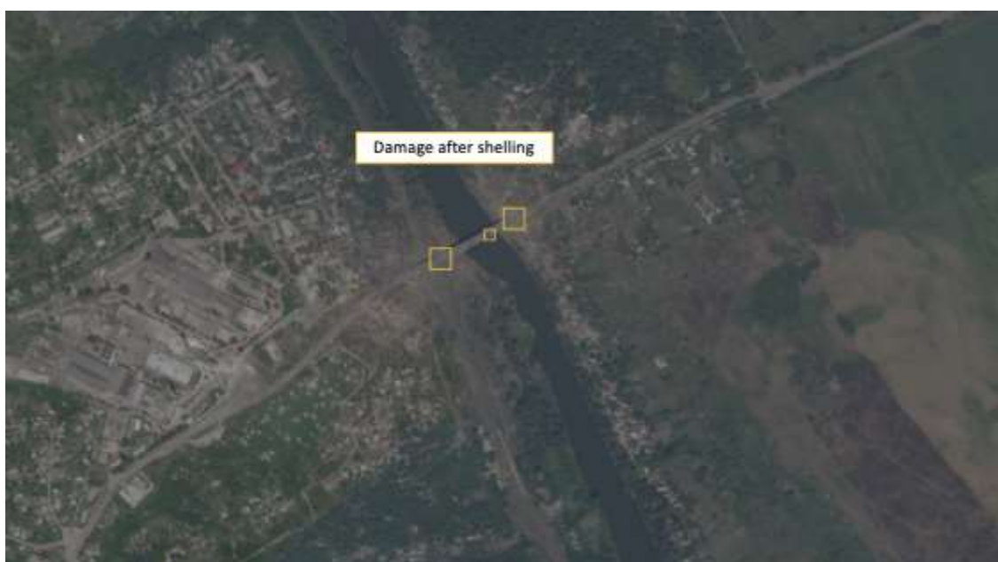
Figure 17: Planet imagery of the P66 Bridge from 19 June, showing damage to the bridge.
